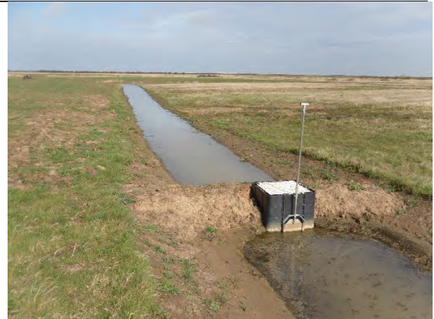
Figure 5b – Scrape with hydraulic control
